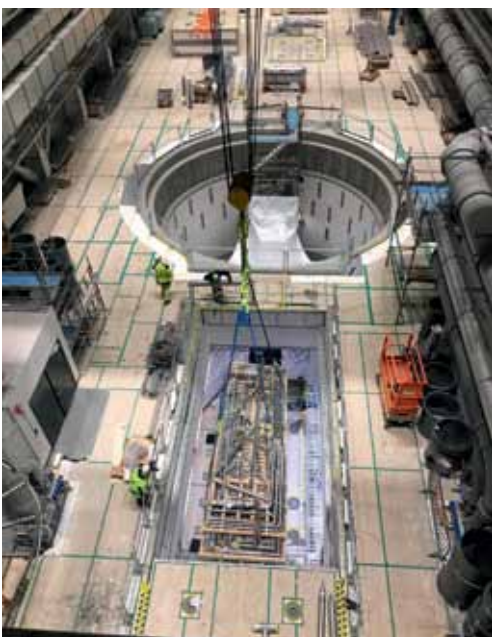
Handling of Demaco's equipment at ESS location.
